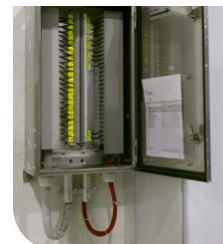
Junction box for terminating field signals and trunk cable
