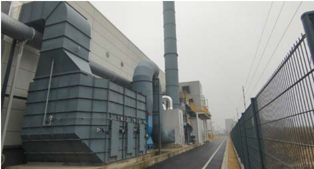
The new painting line's VOC and emission control system has so far achieved an emission reduction of 27 mg/m 3 of the targeted 60 mg/m 3 Chinese standard.
