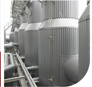
Evaporation plant in Metsä Board's mill in Kaskinen
